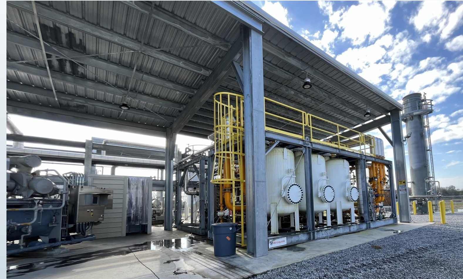
RNG Facility at New River Landfill in Raiford, FL
